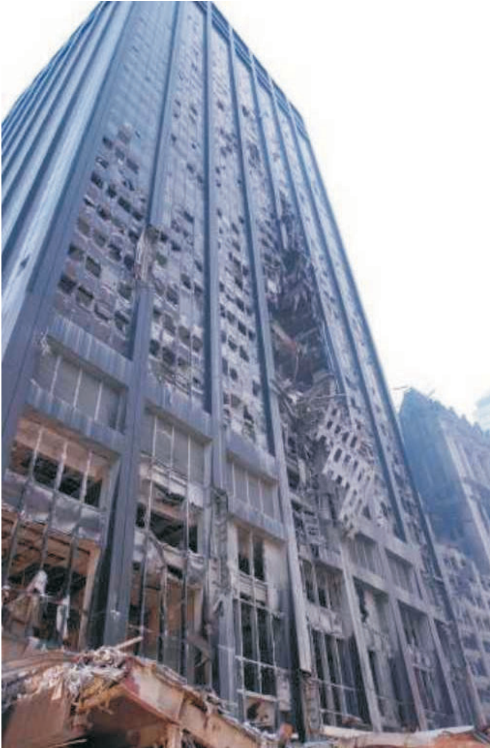
Figure 12-15.—Pyramid form of a destroyed building. (Photo by PHC Eric J. Tilford)
